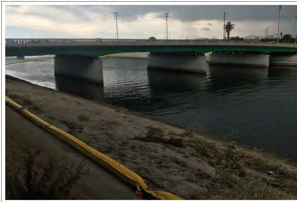
View 9: View looking west from the southern embankment of Ballona Creek at the Lincoln Boulevard Bridge.
