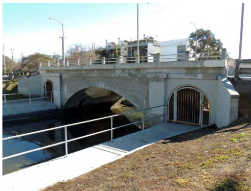
Location: Venice Boulevard over the Grand Canal Name: Pacific Electric Venice Short Line Bridge and Grand Canal Date: 1904
