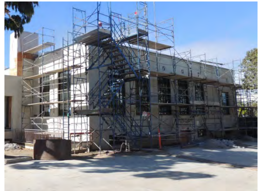
Address: 1601 Main Street Name: Venice Post Office Architect: Louis A. Simon Date: 1939
