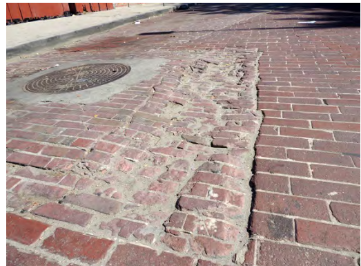
Location: 18 th Avenue between Pacific and Ocean Front Walk Name: 18 th Avenue Brick Street Date: circa 1905
