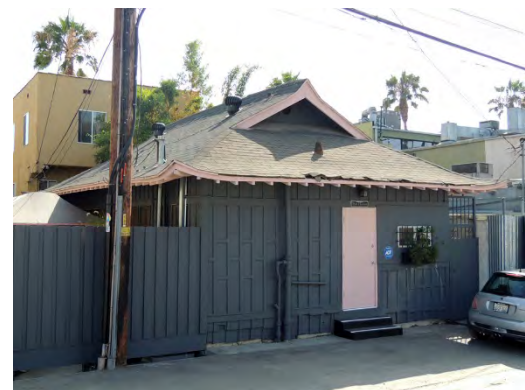
Address: 1641 S. Abbot Kinney Boulevard Name: Pacific Electric Venice Short Line Ticket Building Date: 1911
